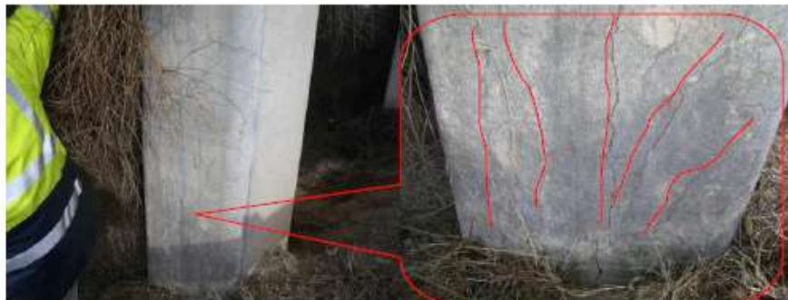
Fig. 5.9 1#Vertical cracks in the body of piers (1)
