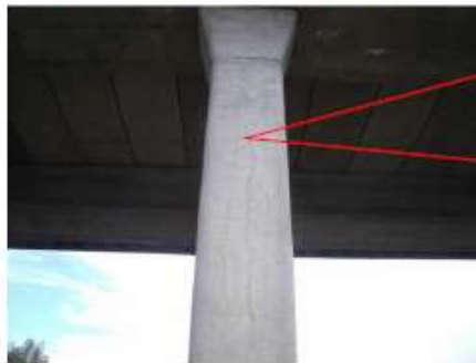
Fig. 5.11 2#the net cracks in the pier body of the bridge pier (1)
